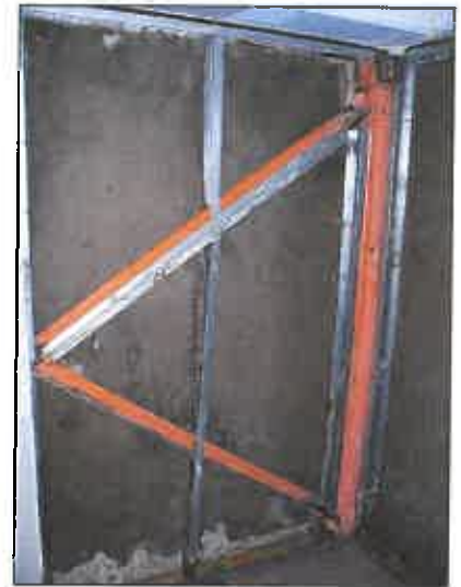
Structural section loss
