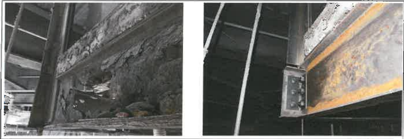
Plaza staircase structural supporting members with holes through the web before repair [left] and after repair [right]
